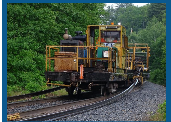
Photo of specialized continuous welded rail train laying new rail on SLR as part of a recent NHDOT project. (SLR photo)
