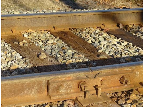
Existing old, bolted rail on SLR mainline. (SLR photo)
